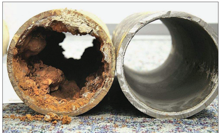
Figure 4: Cut-away of corroded galvanized pipe with rust build-up compared to newer, smooth pipe.
