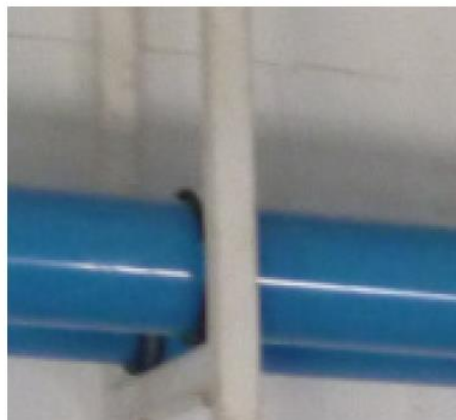
Rigid Pipe Supports from Ceiling
