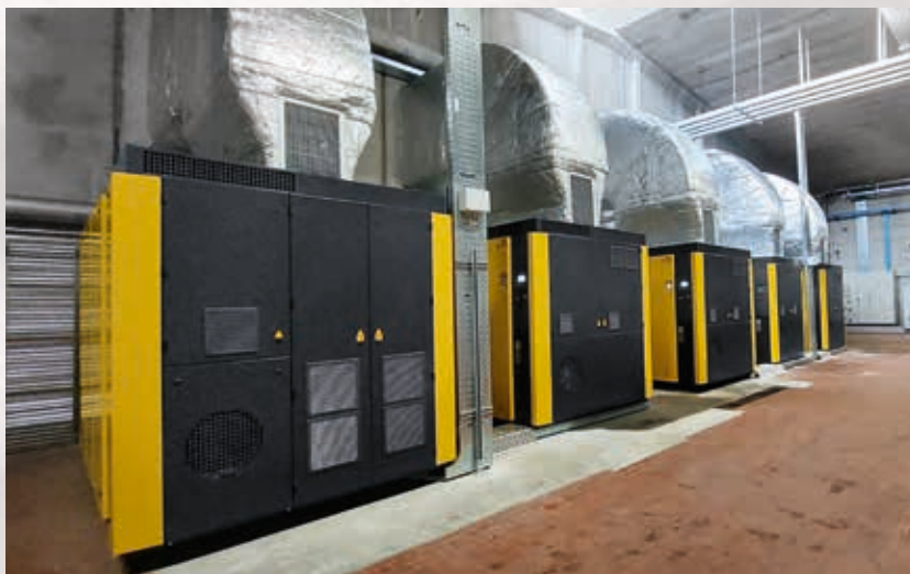
Image left: Cervotessile is renowned for its high-quality products that are rich in traditional history. Image right: The new compressed air station comprises five rotary screw compressors from KAESER.
