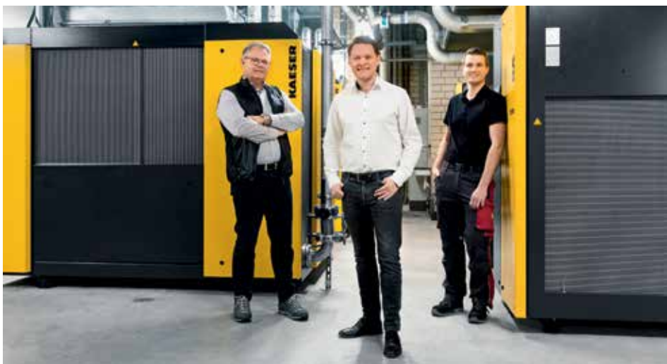
Managing Director Florian Müller-Stauch (centre), Head of Plant Engineering Dirk Brinkmann (left), and Deputy Head of Plant Engineering Yannic Ostermann (right) are delighted with the new compressed air station from KAESER.
