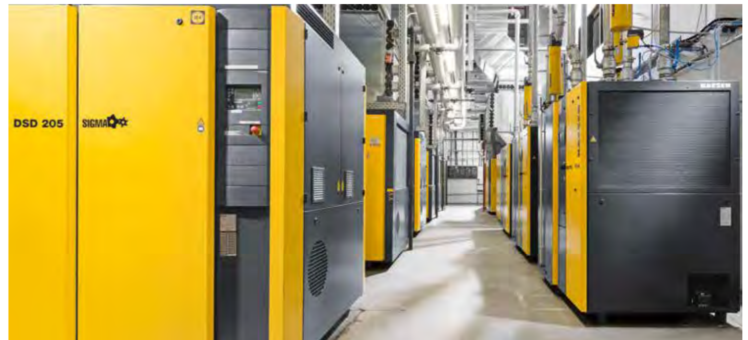
The compressed air production 'Hall of Fame' at nobilia, seen here in plant I.
