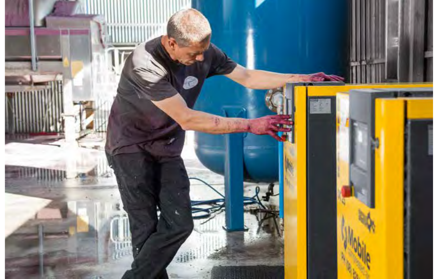
Teusner's new compressed air station: two KAESER SK 25 rotary screw compressors and an air receiver with 1300 gallons of storage capacity.
