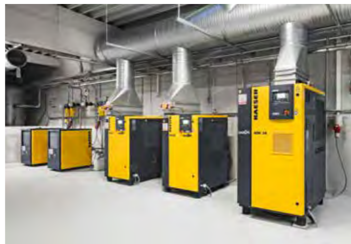
To maintain the required purity class at all times, different sensors transmit their quality parameters to the SIGMA AIR MANAGER 4.0 on a continuous basis.
