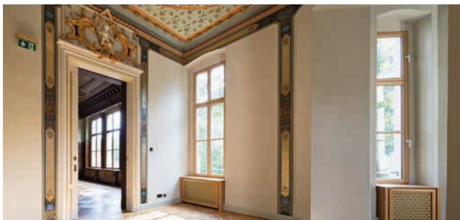
The wooden floor was renovated and partially replaced by a specialty company.
