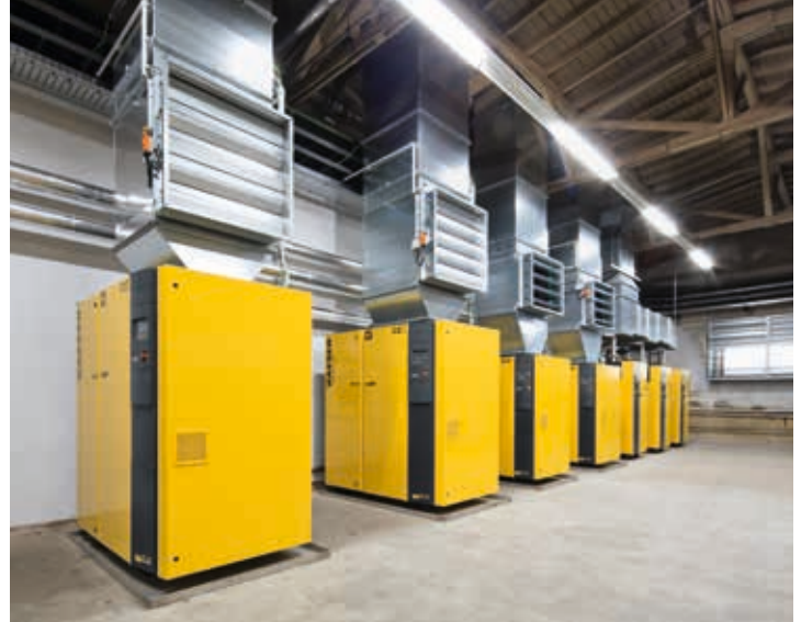
Two KAESER CSD 105 and BSD 75 rotary screw compressors deliver the compressed air for the entire plant.
