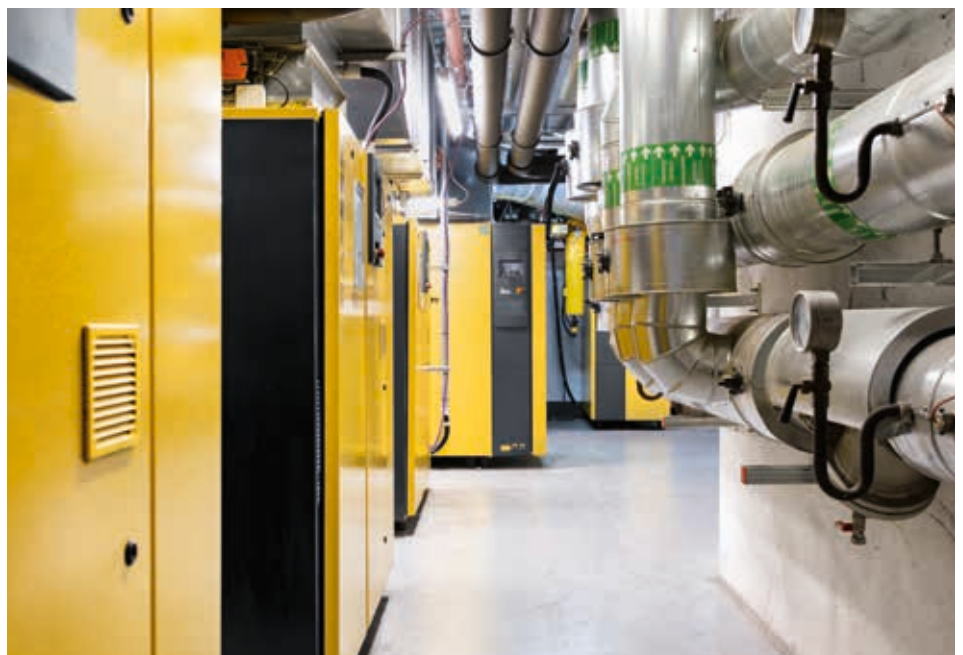
Paving the way for even greater energy savings, the system is already designed for heat recovery in the future.
