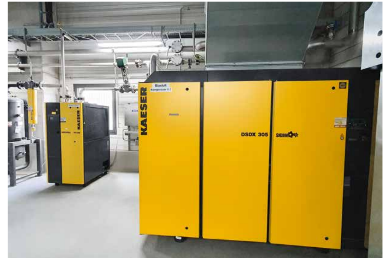
A DSDX 305 rotary screw compressor from KAESER provides blowing air for temporary demand peaks.
