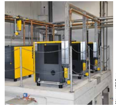
The air system sits high above the production hall, where hot air accumulates, creating high temperatures.
