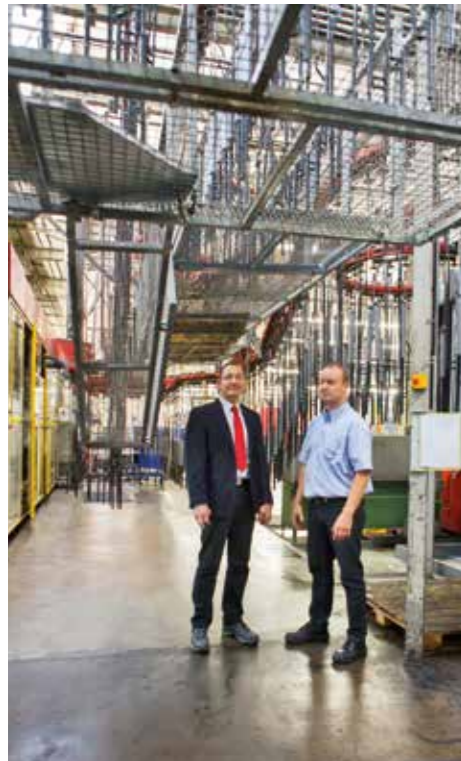
Manuel Baumgarten (ZF Eitorf) on the right and Norbert Hages (KAESER-Bochum branch), left, discuss the significant energy savings delivered thanks to the new air system.
