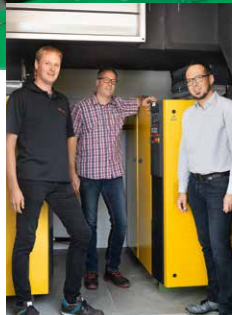
Two KAESER rotary screw compressors ensure maximum energy efficiency for the company's compressed air supply. Deep in discussion (from left to right): Bernd Zimmermann (distributor), Manuel Müller (Richter), Tobias Richter (Richter).
