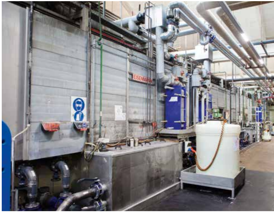
Compressed air plays a key role in the production process at ZF Eitorf.
