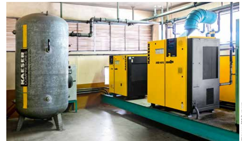
The tailor-made air system for Industria Harinera supplied by KAESER COMPRESORES met – and exceeded – all expectations.
