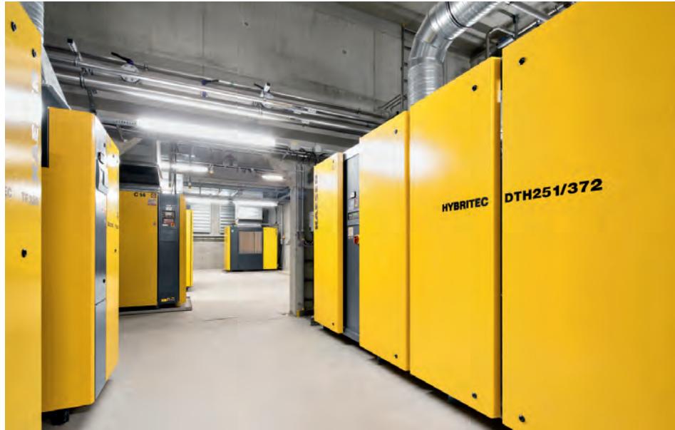
The new compressed air system, which includes a HYBRITEC combination dryer.
