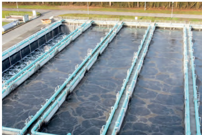
Compressed air is used to supply oxygen for the microorganisms active in the clarification tanks.
