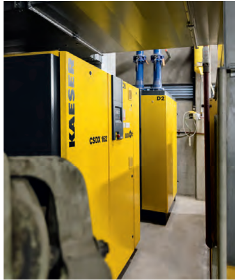
Part of the old compressed air system. It distributes compressed air subject to stringent dryness requirements.
