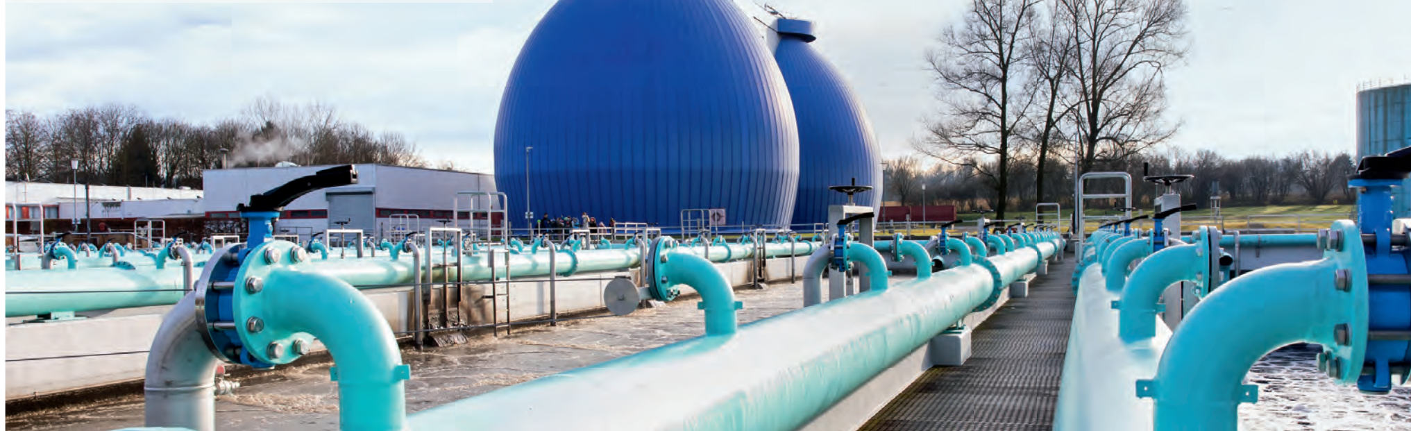
The Langwiese wastewater collection and treatment plant is the largest of its type in the northern catchment area of Lake Constance.
