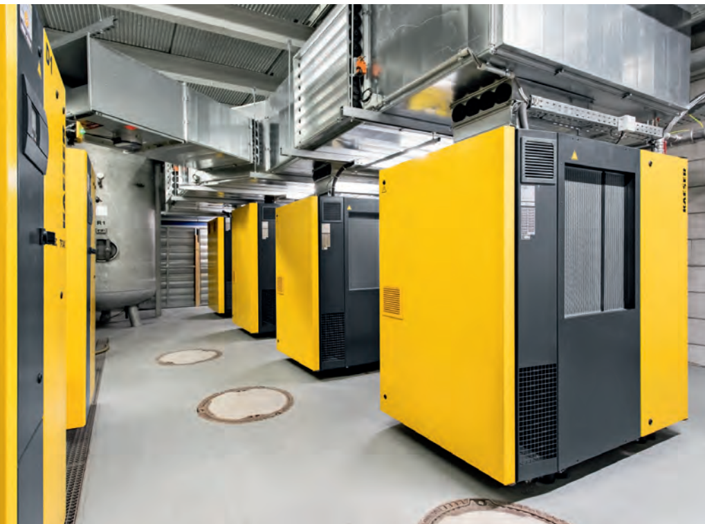
The compressed air station equipped with KAESER rotary screw compressors.
