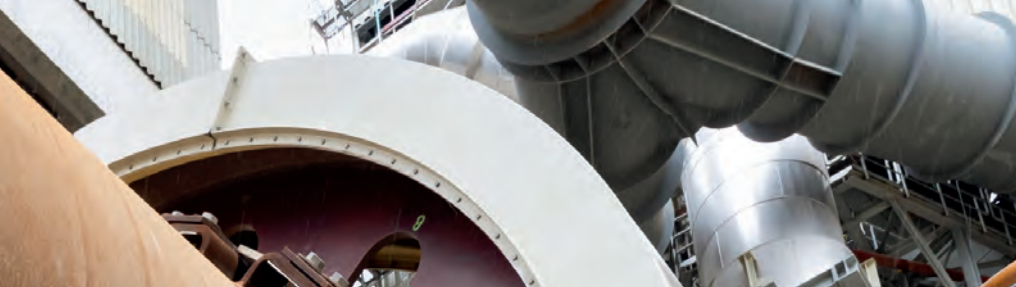
New compressed air system at HeidelbergCement
