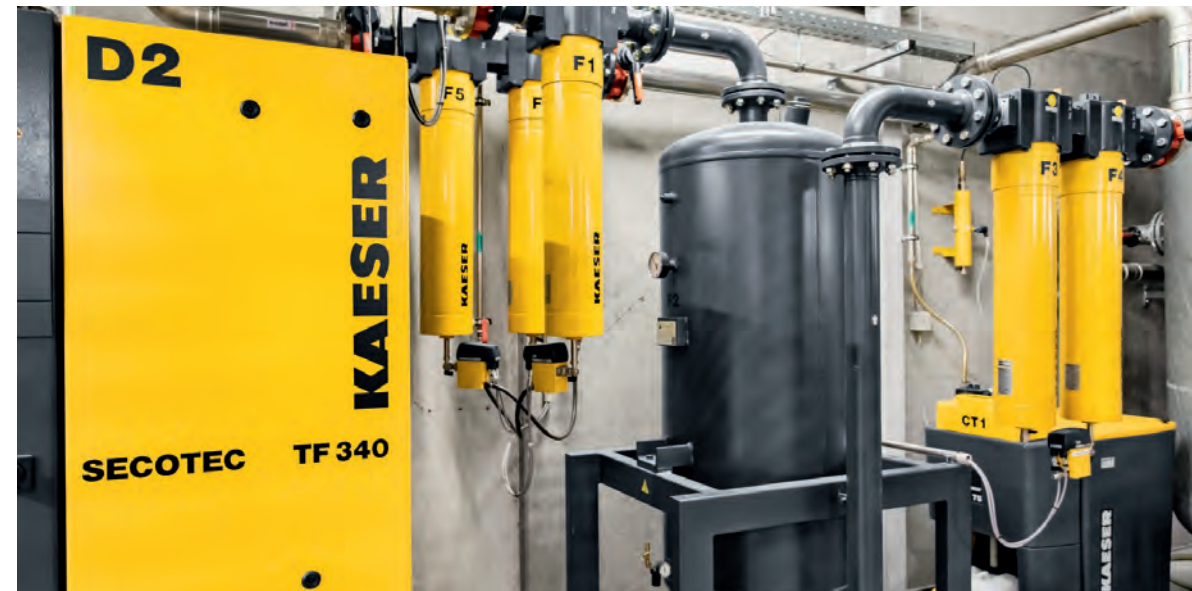
To ensure that the compressed air supply meets the right purity and quality standards, the system includes two TF 340 refrigerated dryers, as well as activated carbon adsorbers and a variety of KAESER filters with very low pressure losses.
