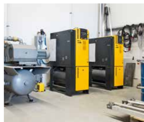
The KAESER station provides the necessary supply of compressed air.
