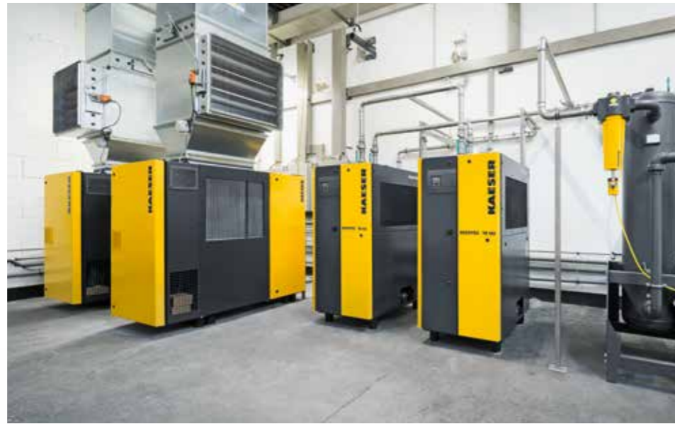
The compressed air supply meets the stringent requirements of Quality Class 1.4.1 in accordance with DIN ISO 8573-1.
