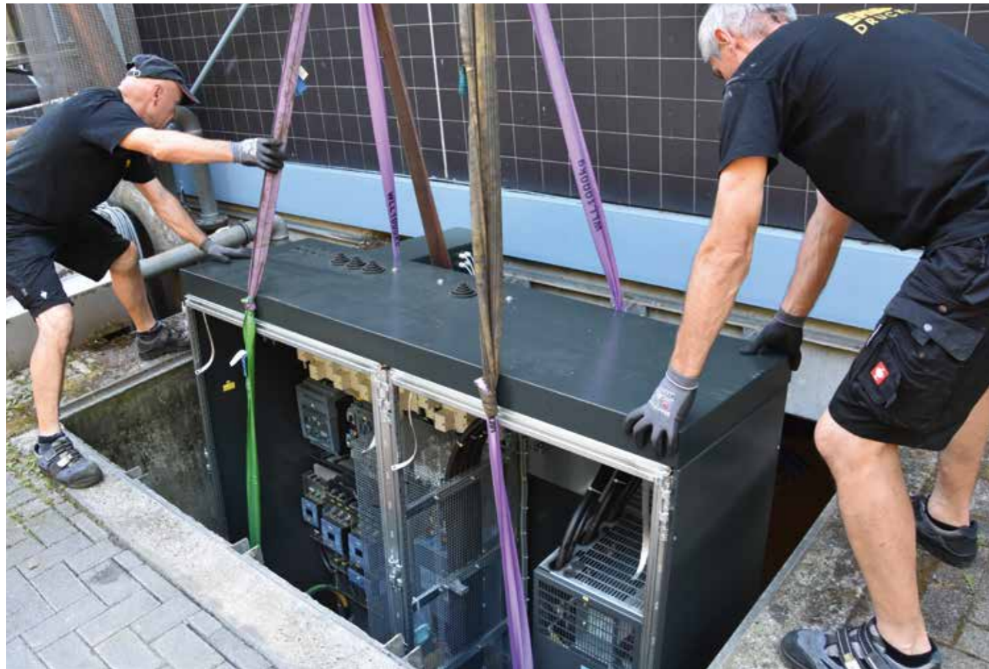
The body of the compressor unit had to be guided carefully through the light shaft.
