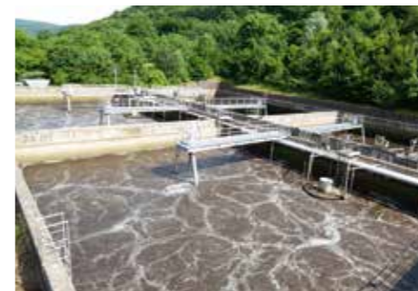
Dependable blower air for supplying oxygen to two aeration tanks
