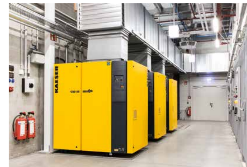
...and the compressed air station in the high-rack warehouse in Distribution Center III, Weiden-Brandweiher
