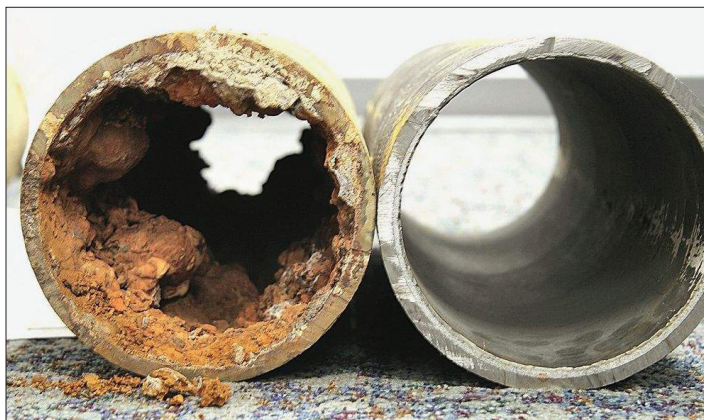
Figure 3: Cut-away of corroded galvanized pipe with rust build-up compared to newer, smooth pipe.
