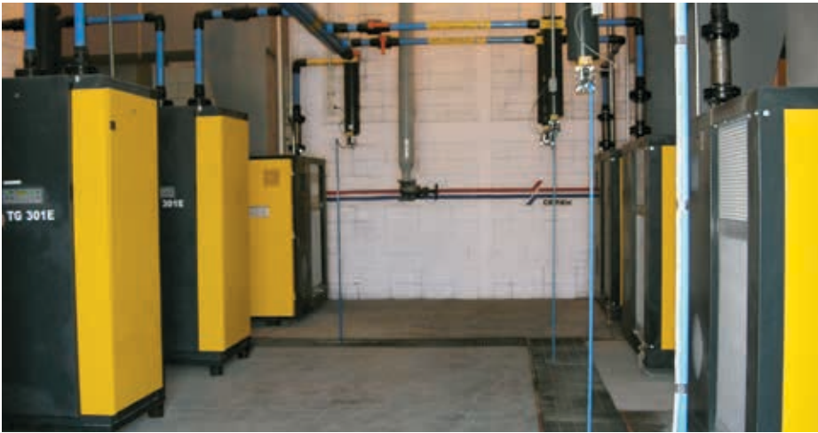
A 2,200 hp indoor installation at a large cement plant.
