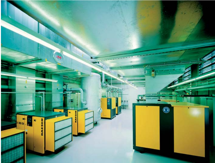
A modern compressed air system with compressor internal controllers and master controllers based on industrial computers at an automotive manufacturer's facility
