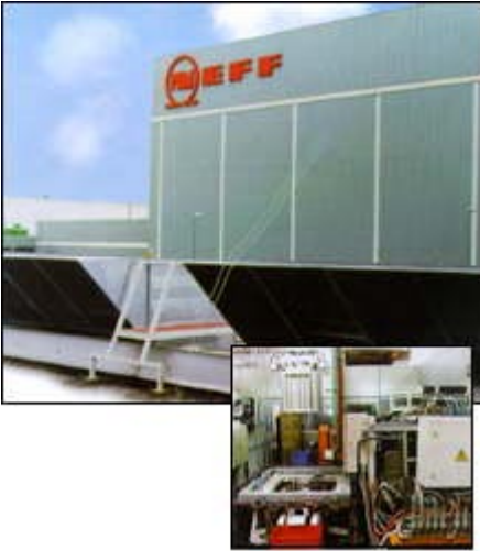
Waste air from compressor cooling is carried away by weatherproof ducting.
